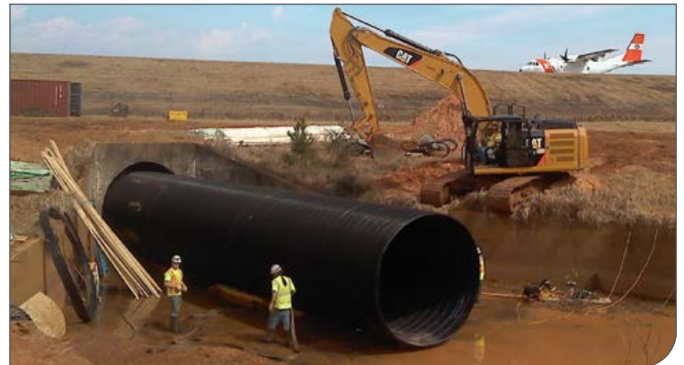
Mobile Regional Airport Runway, AL – segmental sliplining can be installed without interrupting flow line or traffic, providing substantial cost-savings (DuroMaxx® SRPE)
