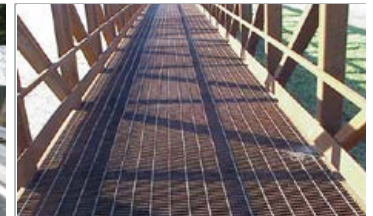
Steel Grate or FRP
