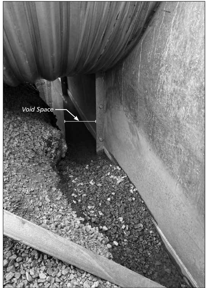
Void space under pipe needs to be filled with aggregate bedding material and compacted.
