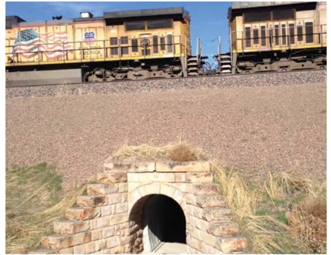
Contech Tunnel Liner Plate was used to fully restore this pedestrian underpass directly under a fully operational rail line.
