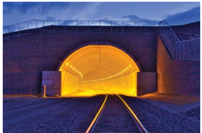
Railway Tunnel – This BEBO structure allowed enough clearance to accommodate the construction of a second railroad track.
