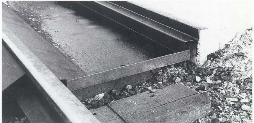
On this installation, concrete platforms were poured with a nosing angle on the edge. A zee flashing angle is welded to the angle, protecting against oil leakage.
