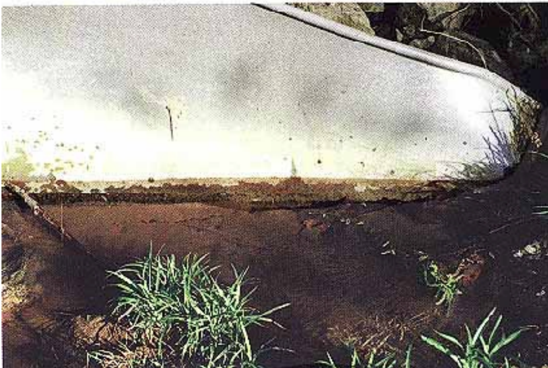
Galvanized End Section (Widely perforated throughout up to waterline - grass growing through)
