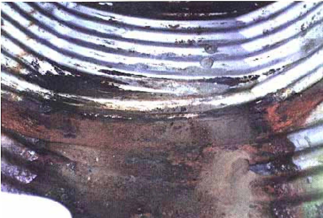
Gwinnett County, GA 10-year-old ALUMINIZED Type 2 pipe and headwall galvanized pipe stub with galvanized coupling band.
