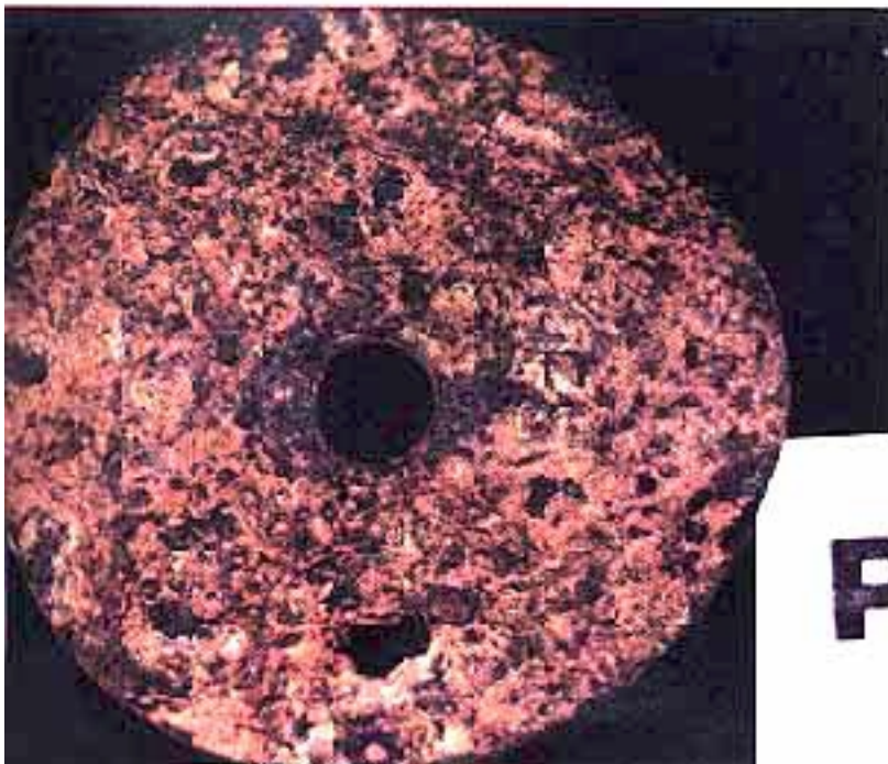
Galvanized Invert - Waterside (Perforated by abrasion)
