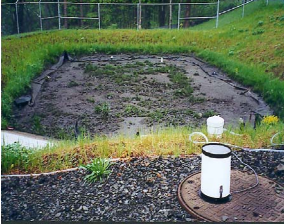
Figure 3: The Sand Filter and rain gage.
