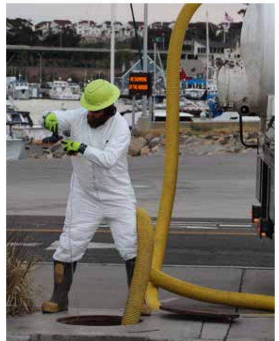
The entire sump of the DSBB is accessible and can be viewed from the finish surface.
