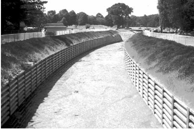
Curved Bin-Walls help achieve drainage area cross-section and protect against bank erosion.
