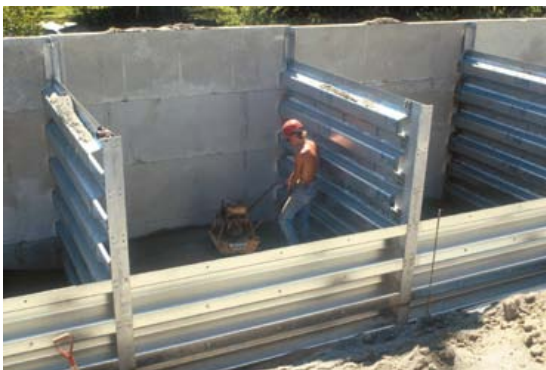
Fill material within and behind the bins should be placed in 4-inch to 8-inch layers and thoroughly compacted with power tampers.
