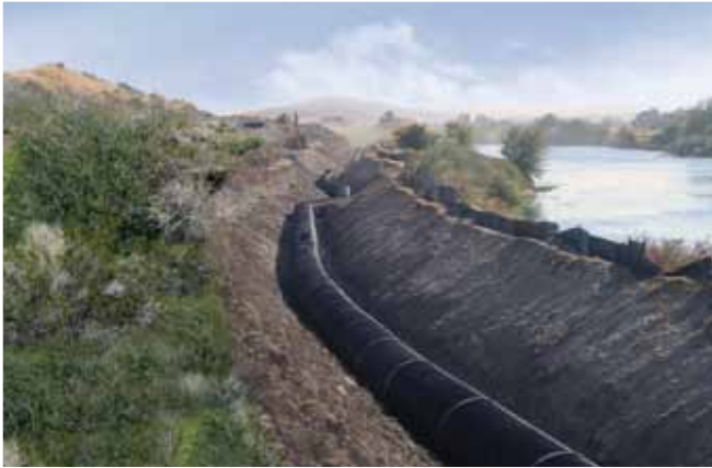
More than three miles of 54" and 60" DuroMaxx SRPE Pipe installed at Barker Ranch.
