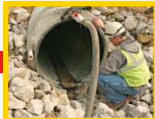
The grout is pumped into the entire length of the pipe, filling in all voids between the new and host pipe, and the areas between the pipe and roadway.
