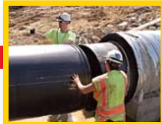
The second piece of pipe is lowered into position, and lined up with the first piece.
