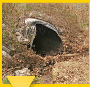
A typical deteriorated culvert close to failure, potentially leading to road collapse and danger to the motoring public.
