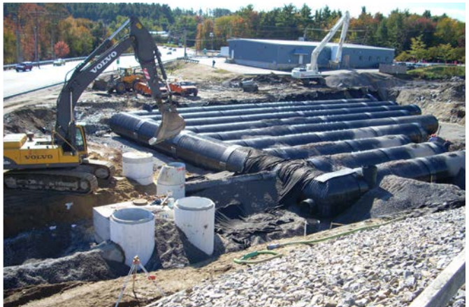
CMP Detention System provides the perfect solution for FAA's requirements to remove any ponded water adjacent to a runway.
