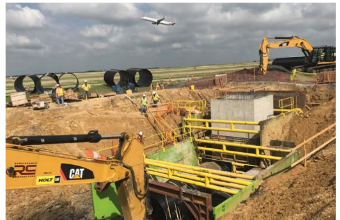
DuroMaxx® SRPE is an extremely efficient solution for glycol storage able to handle the heavy live-loading of an Airbus A380.
