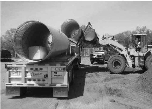
Lifting CMP off the flatbed with a front end loader and forks.
