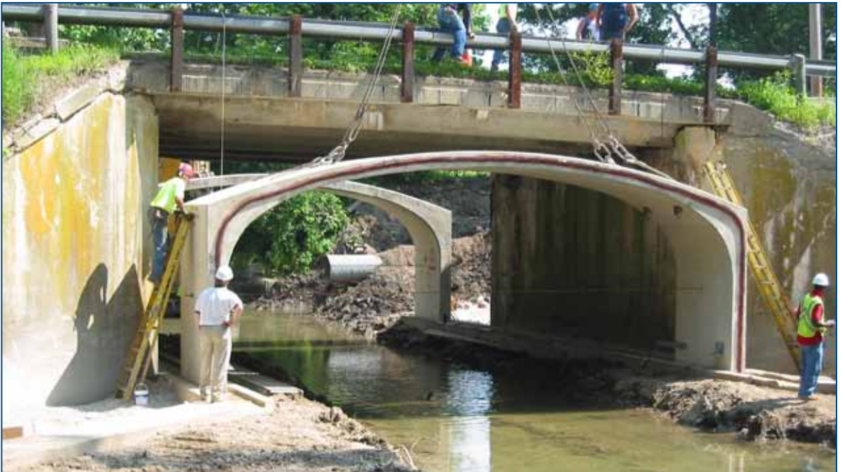
Dayton-Springfield Road (OH) – precast system installed under existing beam bridge to reduce road closure (CON/SPAN)
