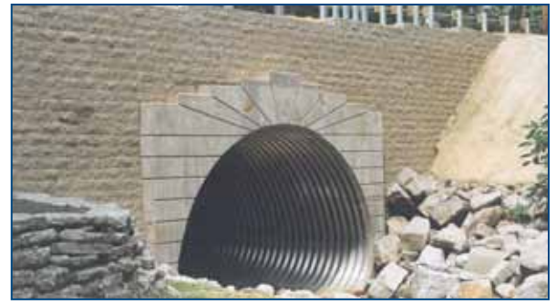
Bath Township (OH) – emergency replacement when flooding washed out a 100-year-old stone arch (ALSP)
