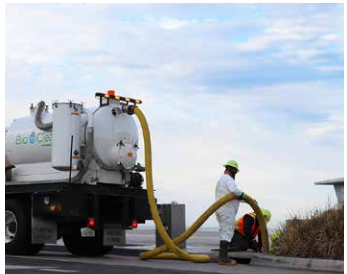
Most Modular Wetland Linear systems can be cleaned in about thirty minutes.
