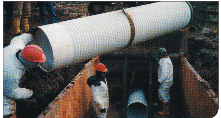
Baltimore Sanitary Sewer, MD – effective segmental sliplining can be installed without interrupting flow line (A2™ Liner)
