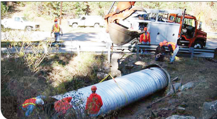
Brook Forest Road Cross Culvert, CO – reline aging culverts to provide exceptional flow and structural integrity (ULTRA FLO®)
