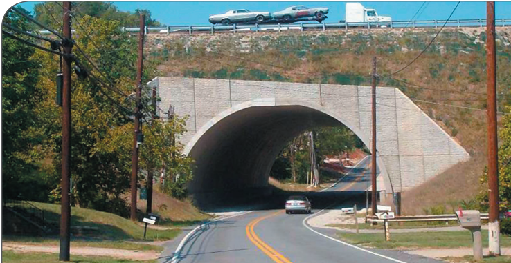
I-64 Huntington, WV – avoid road closures in your rehabilitation efforts with a precast buried bridge (BEBO®)
