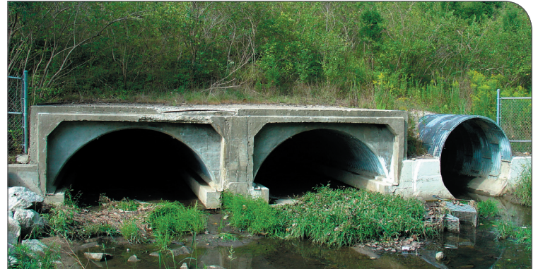
I-675 Culvert Reline, OH – provide optimum shaft stability and protection relining structures under roads (Tunnel Liner Plate)
