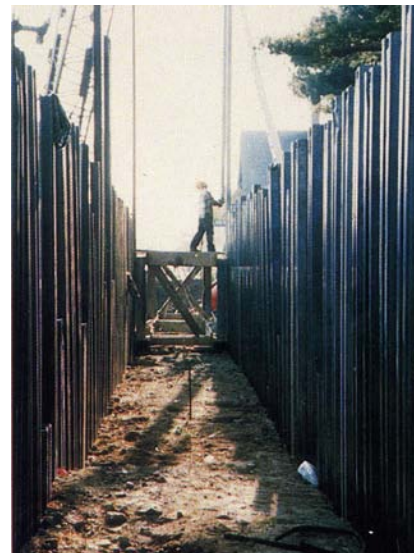
Twin rows of Contech Metric Sheeting used as trench shoring. Increased stiffness means that lighter than normal gages of sheeting can be used.
