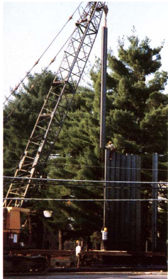
Long sections of Contech Metric Sheeting will be used as trench shoring for this sanitary sewer installation in New York.
