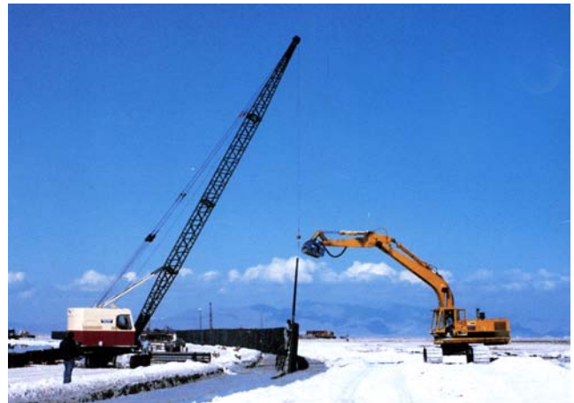
Steel cut-off wall located on a large minerals mine site formed with Contech Metric Sheeting.
