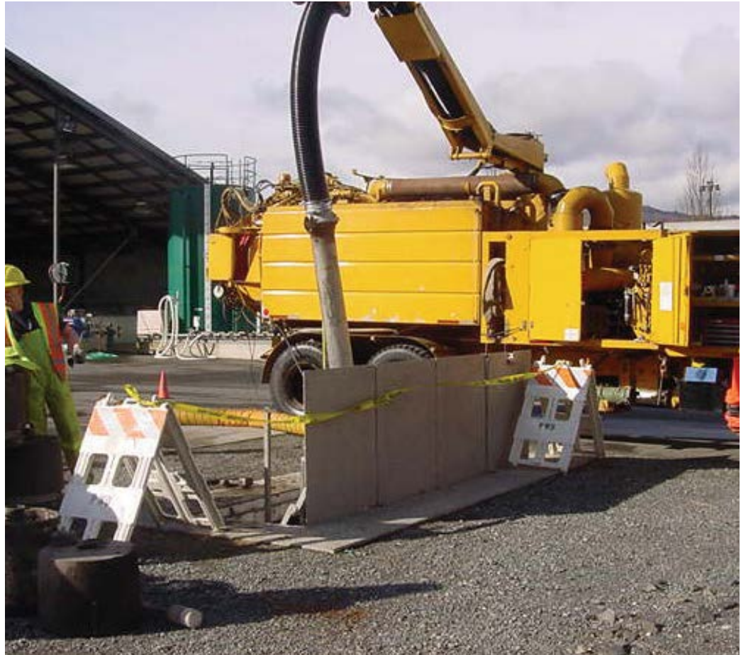
An easy-to-access treatment system can make all the difference in maintenance expenses.
