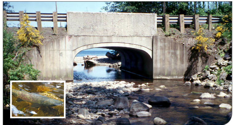
Wild Salmon Passage – a single span, three-sided structure replaces high velocity culverts to provide ideal natural conditions for fish passage and habitat
